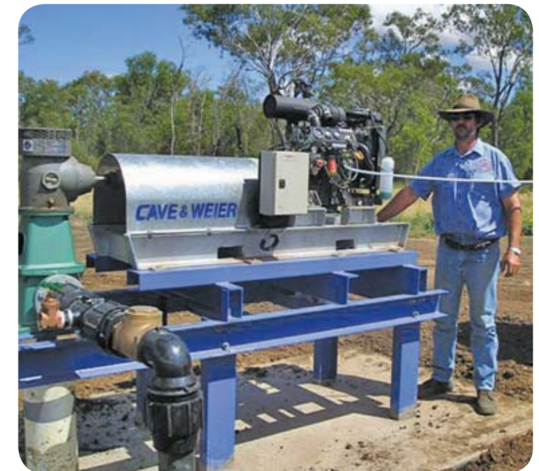
Jeff Weier from McCrackens, Cave and Weier Water Services standing alongside one of the Yanmar powered bore hole pumps
