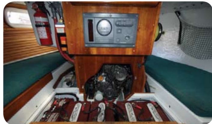
The Yanmar 1GM10C engine neatly installed in Velella
