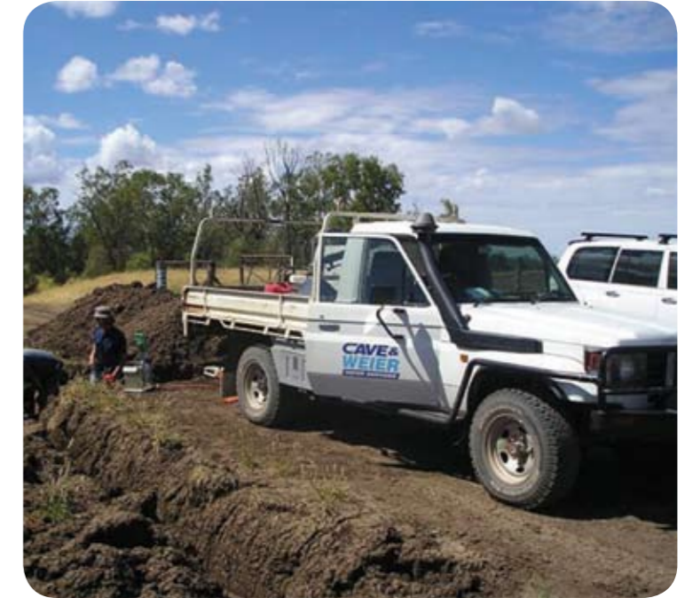
Over 5 kilometers of trenches were excavated to house enough pipe to supply bore water to 10,000 head of cattle
